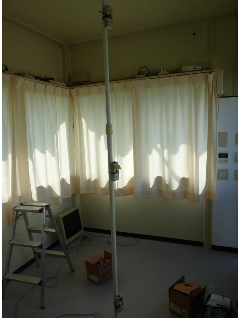
Figure 5.3: three temperature Humidity server in TANS2A
