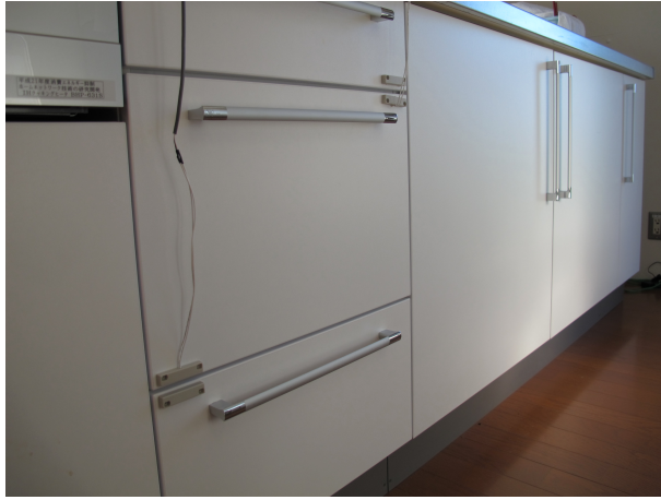
Figure 4.6: The “Cupboard” with magnetic sensor
