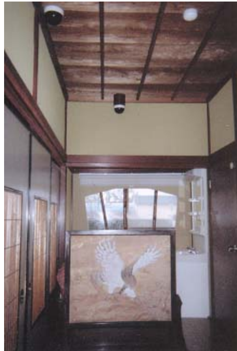
Fig. 1. Two cameras installed in the entrance hall
